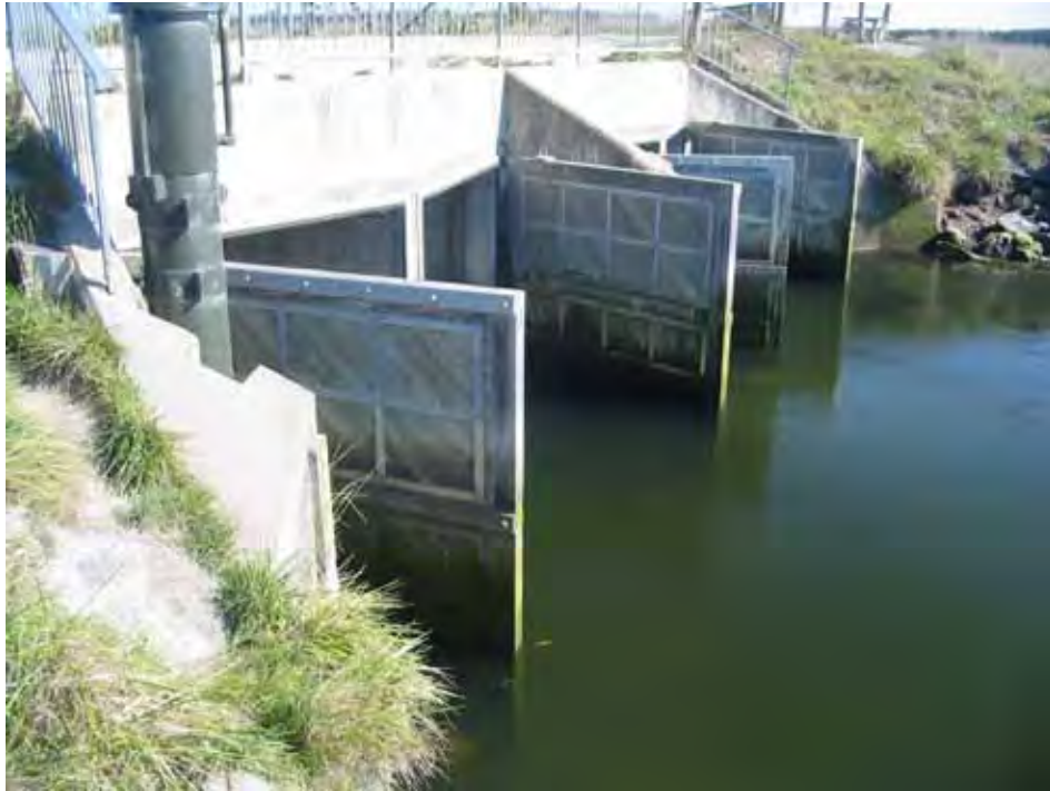
Figure 1. The tidegates on the lower Styx River, pushed open by the falling tide.
