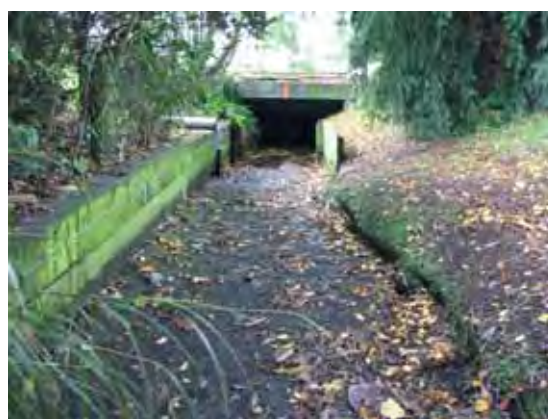
Figure 19. The upstream end of the Kaputone Stream culvert under the Main North Road on 16 May.
