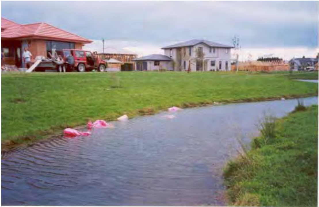
Figure 7. Pink fibreglass insulation material (and its wrapping) has blown into the waterway from adjacent building sites. Upon request, this rubbish was removed by contractors.
