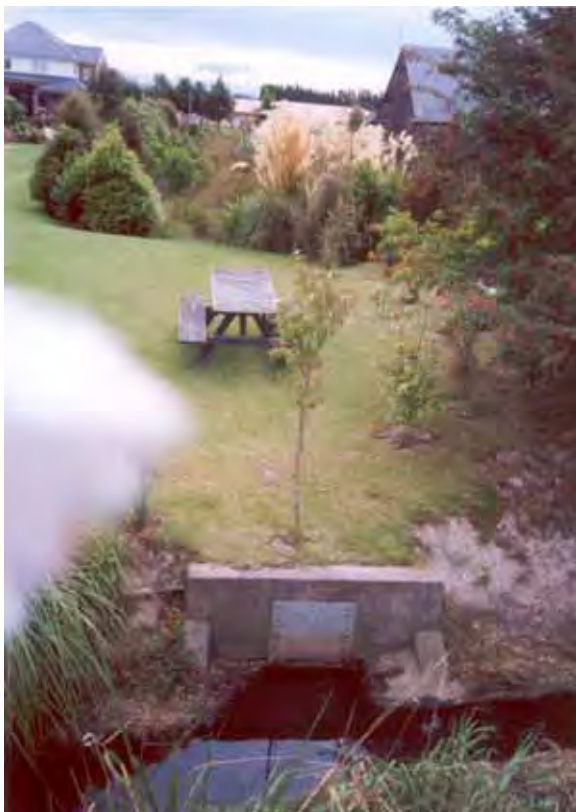
Figure 2. The concrete intake which diverts flow through a pipe (under the garden seat) into the vegetated channel in the background.
